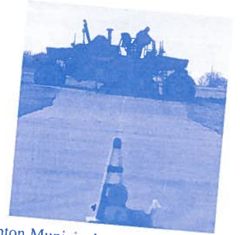
Denton Municipal Airport - some of the taxiways from the airport hangar area are closed as a new taxiway is currently under construction. City officials recently approved a bid for the design and construction of the airport's first control tower.
