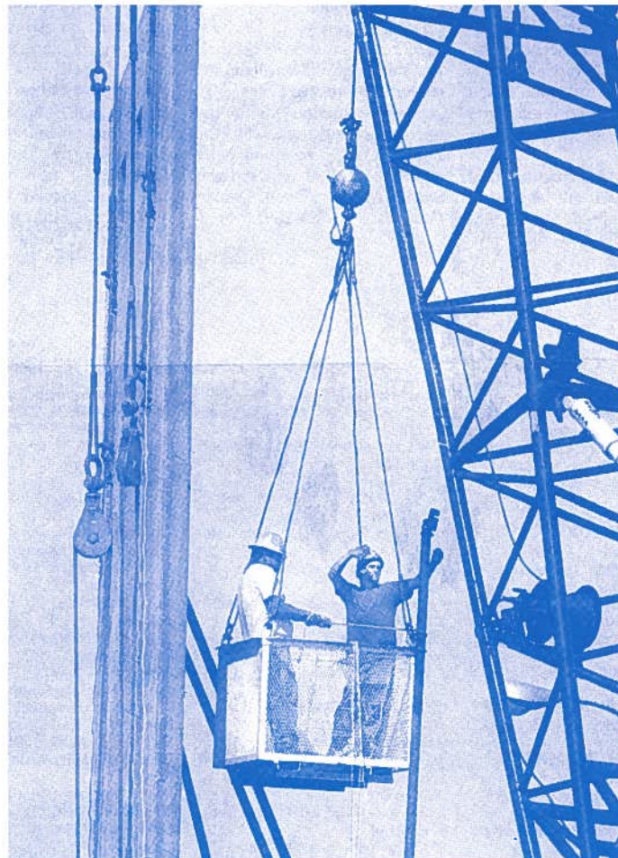
DENTON MUNICIPAL AIRPORT - Workers were lifted up this summer to put the supports on the first wall of the new control tower. The tower is now in place and in operation.
