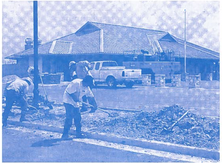
Brenham Municipal Airport - Recent rains did not slow down the work this summer as contractors spread dirt around the median in the parking lot of the new airport terminal.
